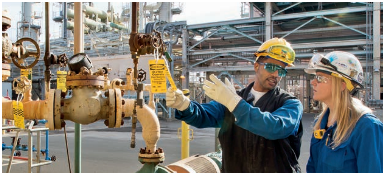
Photo: Two Chevron colleagues review valve tags during a field walk in the alkylation unit at our Richmond Refinery in Richmond, California. Our workforce is dedicated to delivering value through safe and reliable performance by managing the integrity of our equipment and operating systems.
