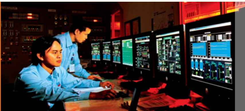
Iskandar Haryanto (seated) and Nanang Nurjaman, production operators at Chevron's geothermal plant in Salak, West Java, Indonesia, monitor the overall plant operations from the control room.
