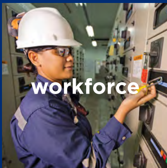
Worker checks a control panel in a substation at Oronite's additive manufacturing plant on Jurong Island, Singapore.
