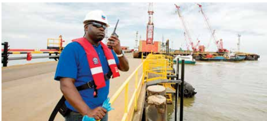
Everyone at Chevron in Angola has the responsibility to use Stop Work Authority if a potentially unsafe situation is observed.
